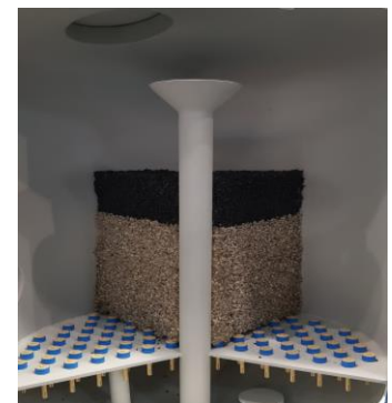
Inside of the GRP Tank
